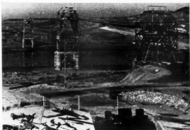
CABLEWAY. —This new installation with capacity of 23 tons was built by I.P.C. over the Tigris River. It replaces ferries and a lighter cableway used previously.
